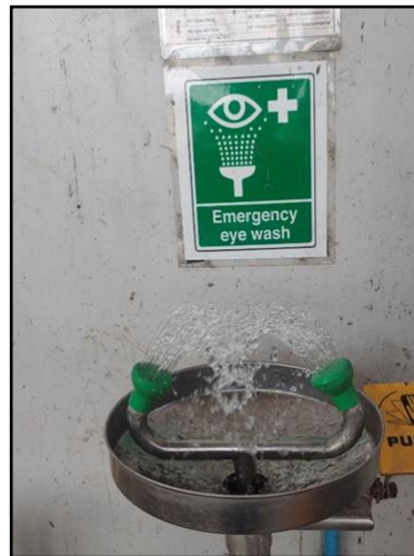
Eyewash station inspection and testing.
