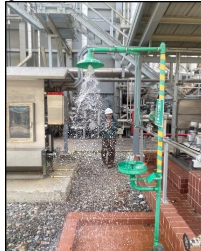
Eyewash shower station inspection and testing.
