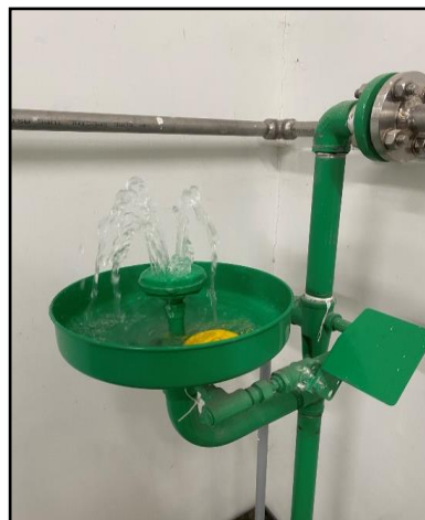
Eyewash station inspection and testing.
