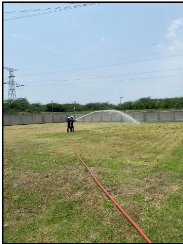
Fire hydrant and hose inspection and testing
