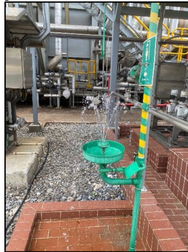
Eyewash shower station inspection and testing.
